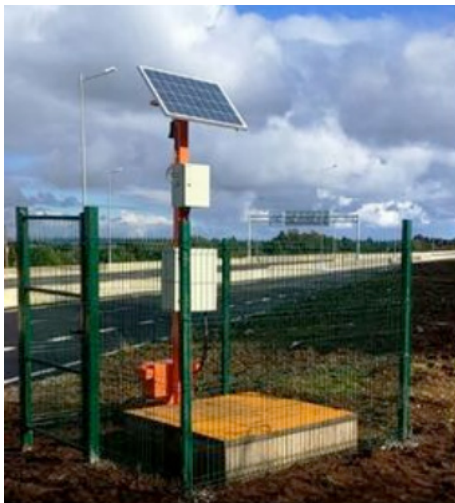
Typical solar power installation
