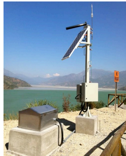
Typical solar power installation including lightning protection system
