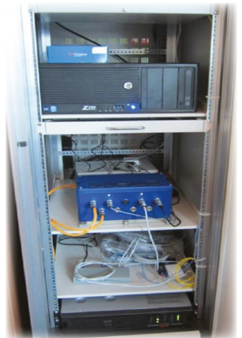
GMSplus6 data logger and PC storage at base point.
