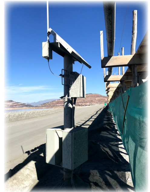
The main wall and west wall of the tailings dam are continually monitored.
