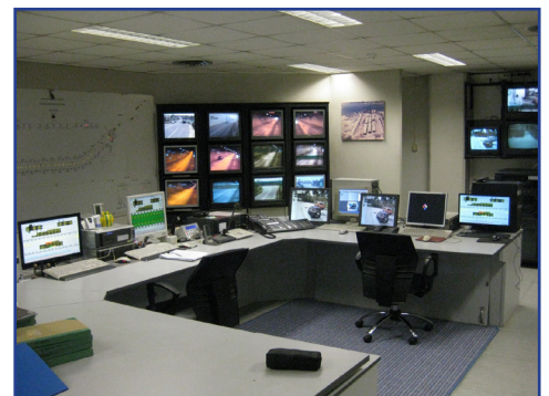
The tunnel is monitored by this control center in Preveza.
