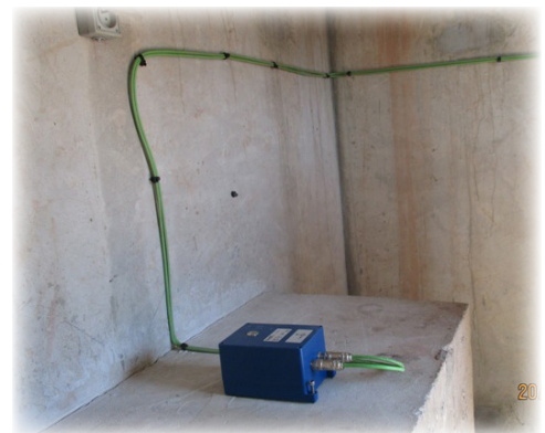
Triaxial force balance accelerometer, AC-73D, in situ.
