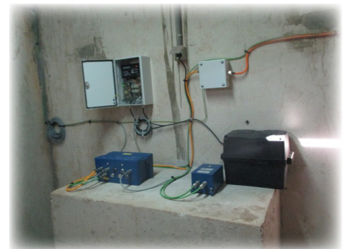
GeoSIG instruments at the seismic monitoring station at My Hassan 1st Dam.
