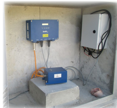
Martil Dam seismic monitoring station
