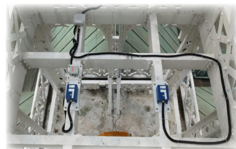
Sensors installed at Angelus Dei Tower
