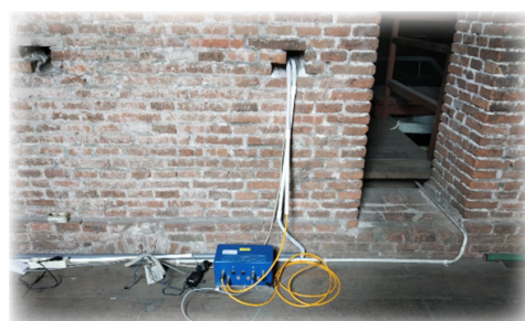
GMSplus6 data loggers are installed in the cathedral's attic and at ground floor.
