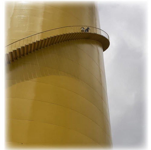
Andalan Tunas Mandiri's crew faced high winds while climbing the 58m surge tank.
