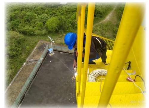
Engineers had quite a view while installing the cabling for the project.
