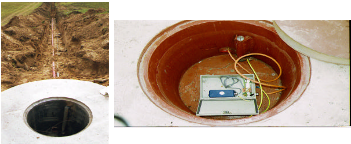
Fig. 4 Photograph of seismic substation (left: substation with 500 m long cable trench to seismic station; right: instrumentation of seismic substation)
